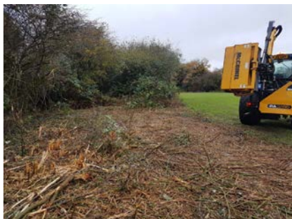
Clearance of site for new pavilion to undertake soil and foundation tests
