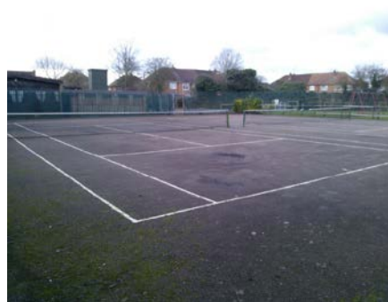
Sub-standard surface at tennis courts
