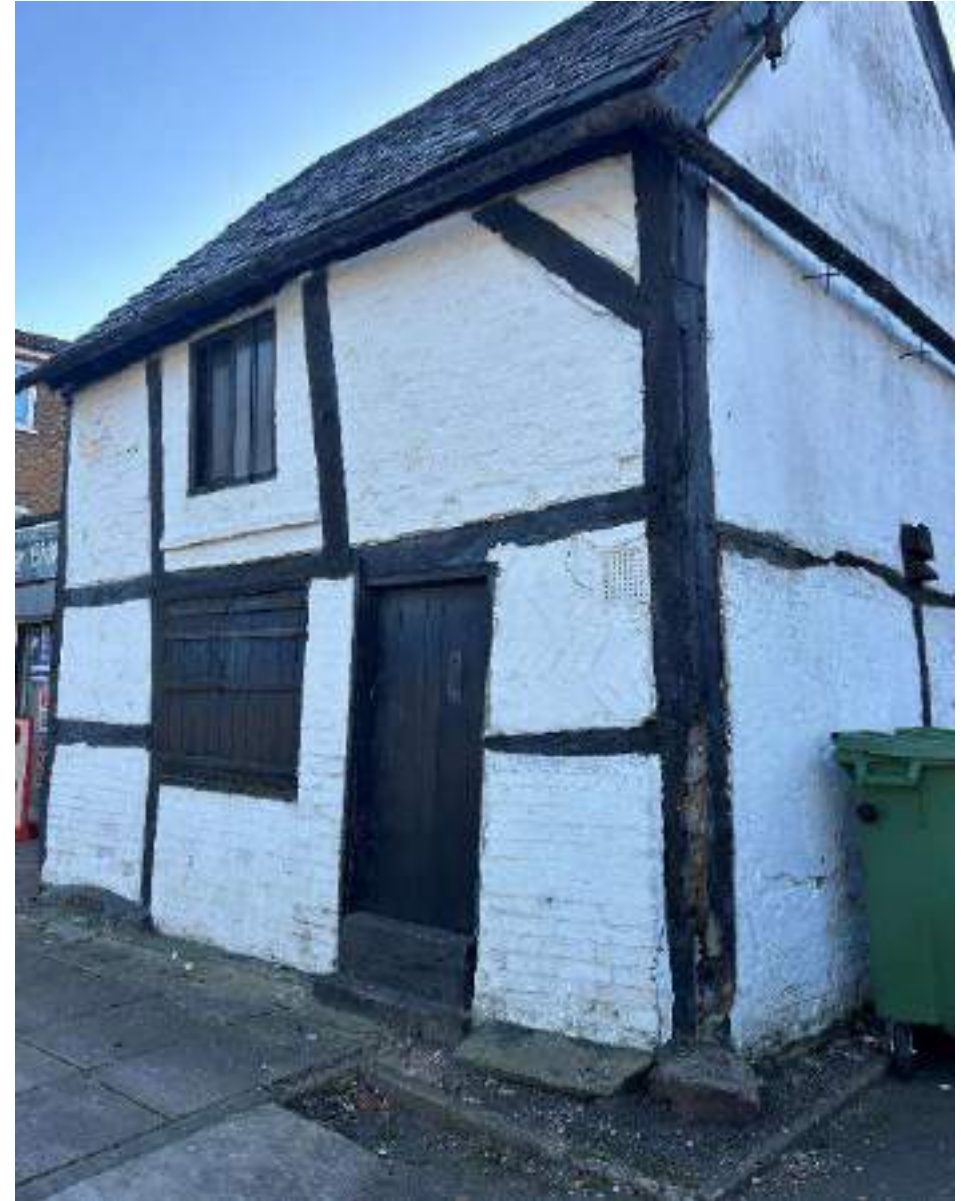
Image 19: Traditional materials use in the building with less cohesive floorscape materials below the plinth.
