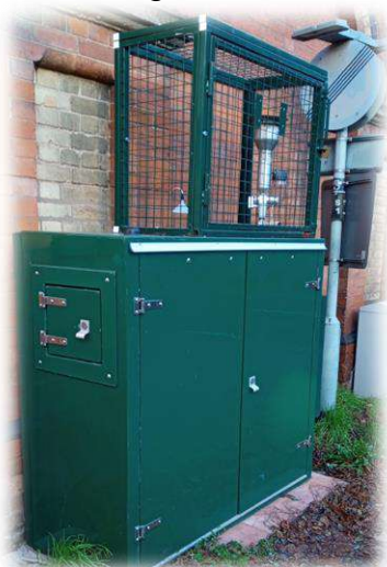
Air Quality Monitoring Station
